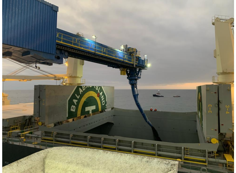
Ship loader in South America – Level 3 FAM ACS under engineering phase
